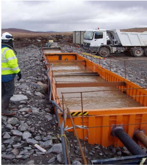
Figure 10-2 Settlement Tanks [Source SEPA Engineering in the Water Environment Good Practice Guide Temporary Construction Methods]
